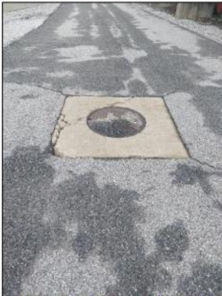
Photo 3: View of Cracked MH Cover Collar
