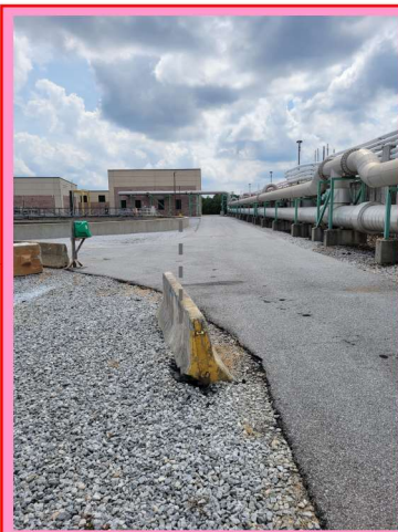
SAWCUT EXISTING DRIVEWAY PAVEMENT USING WIDER ROAD SECTION AS LIMIT OF CUT.
