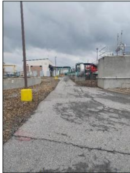
Photo 2: View of Pavement near Secondary Clarifiers
