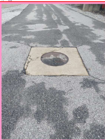
REMOVE AND REPLACE EXISTING CONCRETE COLLAR AROUND MANHOLE TOP. SEE MANHOLE COLLAR DETAIL.
