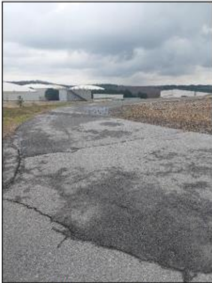
Photo 1: View of Pavement near Secondary Clarifiers
