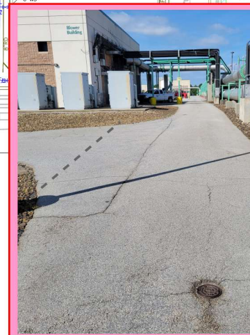
ADJUST WATER VALVE BOX TOP TO MATCH EXISTING VALVE ELEVATION. ADJUST EXISTING VALVE BOX HEIGHT WITH A RISER RING AS MANUFACTURED BY EJ COMPANY. SAWCUT INTO DRIVEWAY TO REMOVE EXISTING JOINT.
