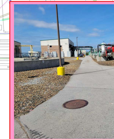
MILL AND REPLACE TO MATCH NEW PAVEMENT TO EXISTING MANHOLE COVER ELEVATION.
