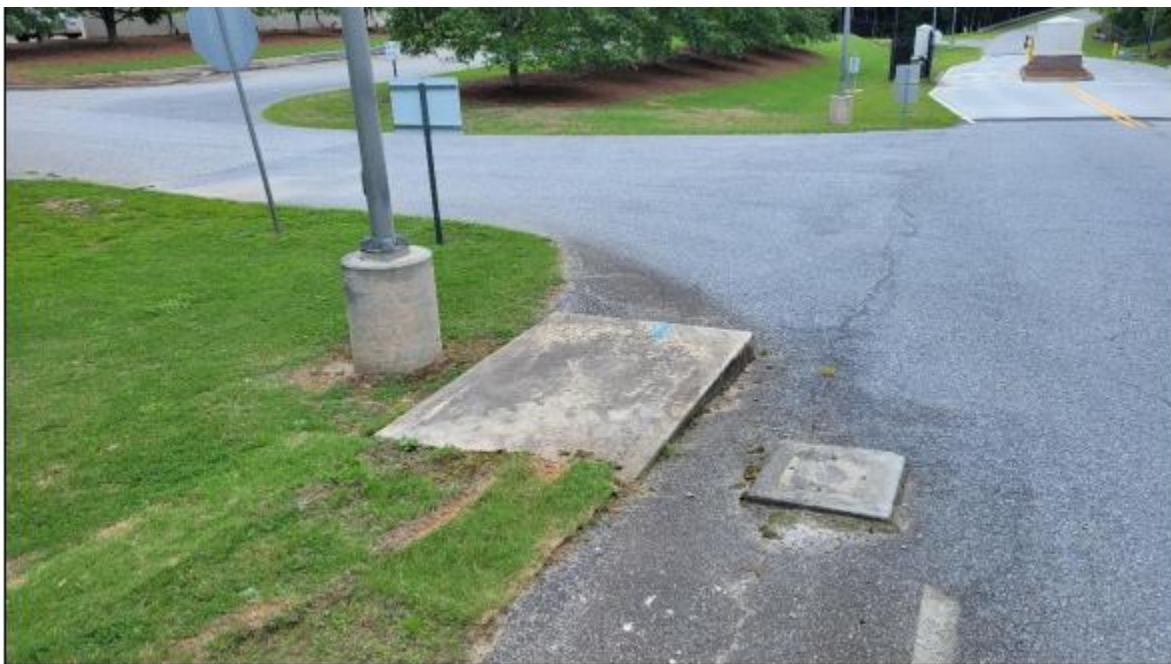
Photo 7: Two abandoned concrete pads to be removed and restored.
