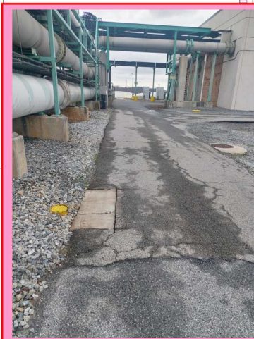
REMOVE EXISTING CONCRETE PATCH. SAWCUT 2'-0" INSIDE OF PATCH AND RECONNECT. REPAVE WITH ASPHALT PAVEMENT AS PER THE PAVEMENT CONNECTION DETAIL.
